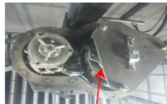
Unguarded Bridge Crane Brake
